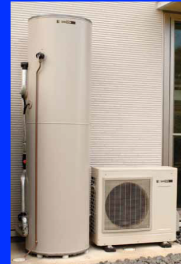
Heat pump hot water
